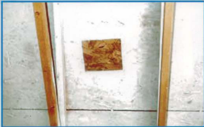
Photograph of roof deck sprayed with HeatBloc-Ultra with a small square area left exposed.
